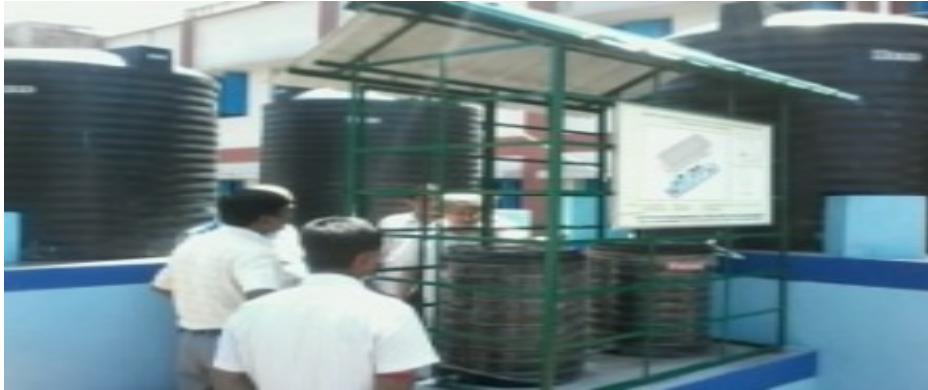
RAIN WATER HARVESTING PLANT
