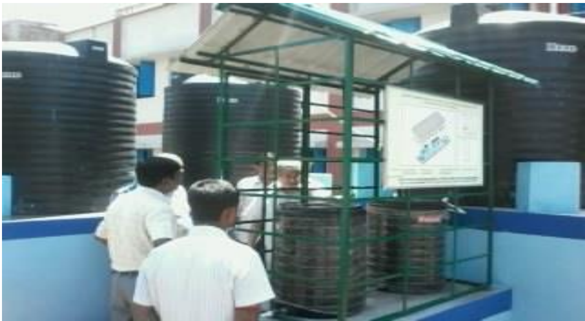
RAIN WATER HARVESTING PLANT, 2016.
